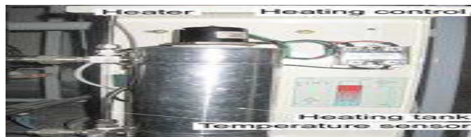
Figure 2: Temperature Control System
